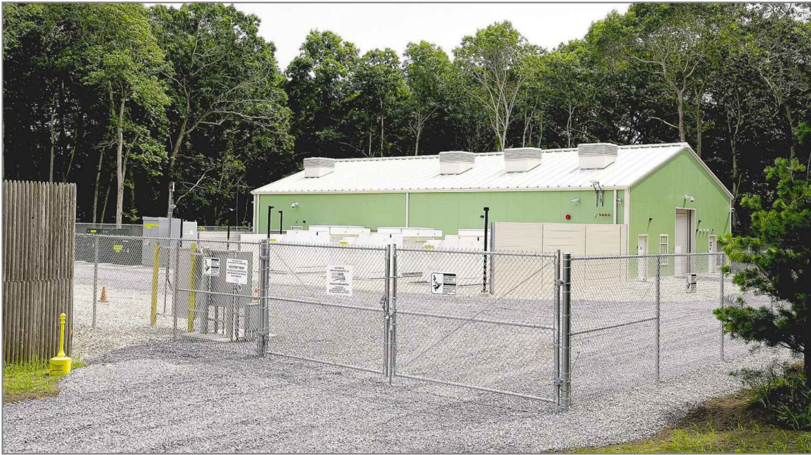
The a 5-megawatt battery plant in East Hampton had a May 31 fire that will keep the facility out of operation until June, officials say.
